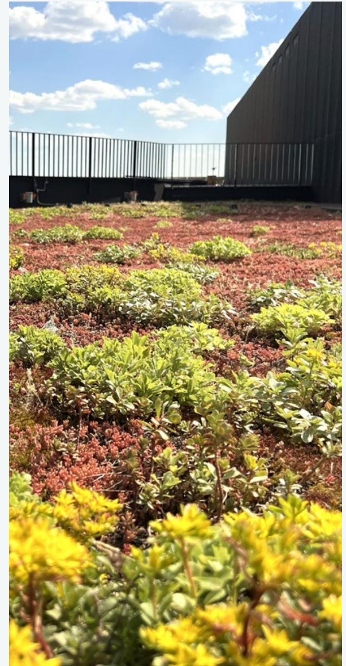
Beautiful sedum roof at the Nowy Rynek D property in Poznan, Poland.
